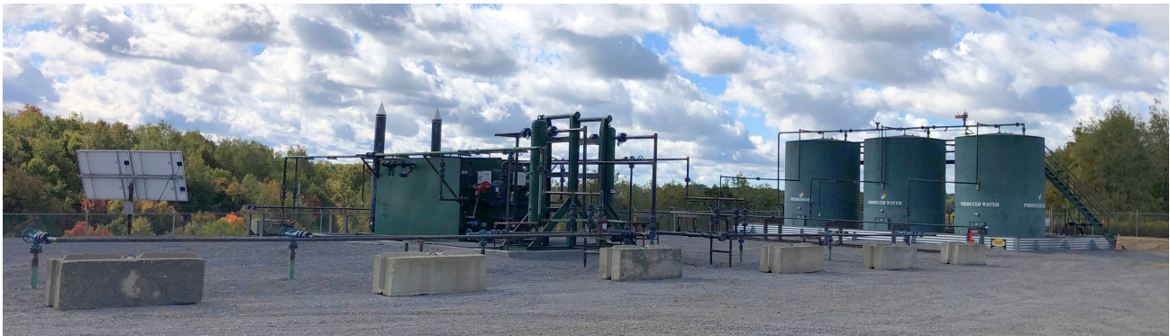
After: The same acquired facility after a full modification project, which enhanced its environmental and safety profile.
